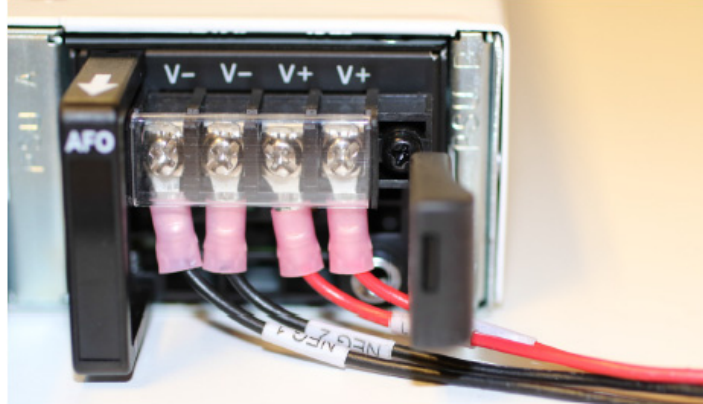
Figure 30 DC terminal block
